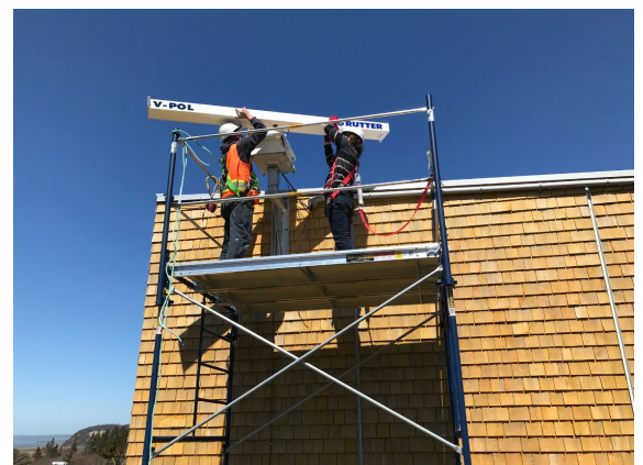
Radar MkII installation at FORCE VC in April
