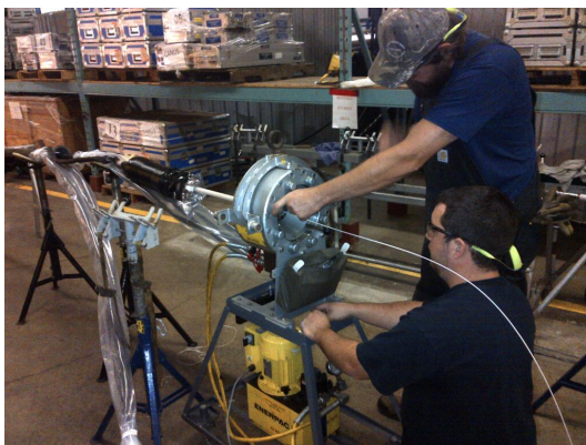
Data cable: fitting abandonment termination that will allow connection with subsea monitoring platform.
